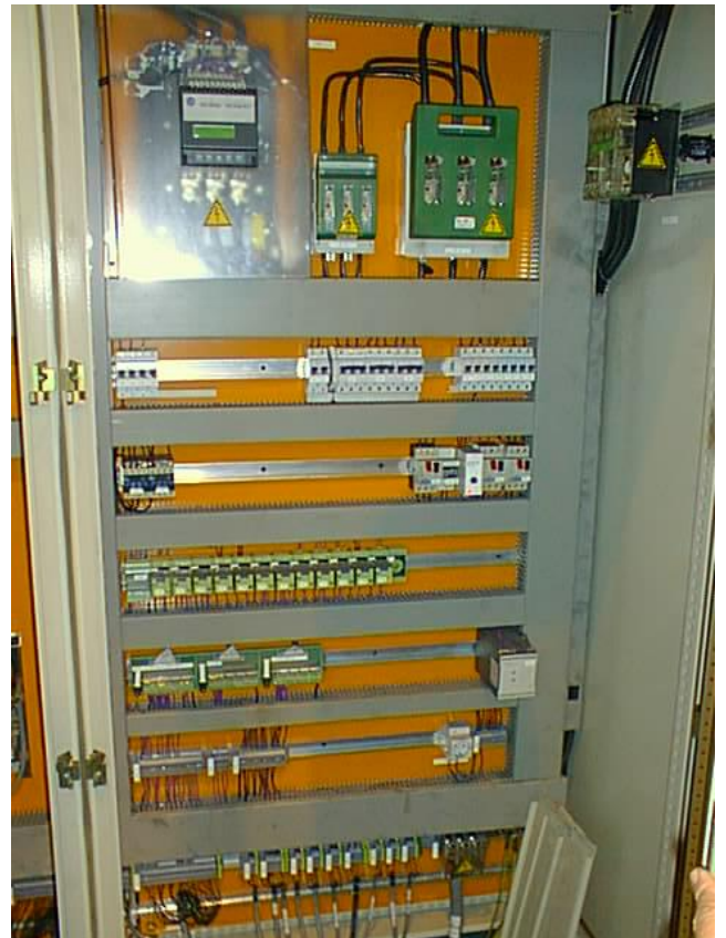
Figure 11: The whole electrical system was completely renewed, according to the provisions of the final customer.
