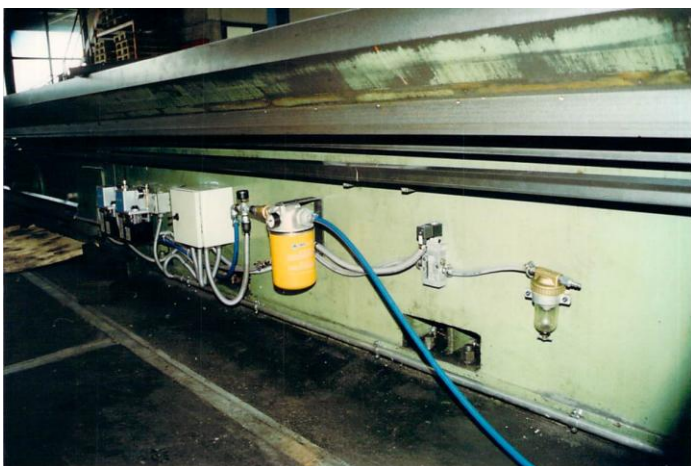
Figure 6: The feed with a filtration, and the control box.
