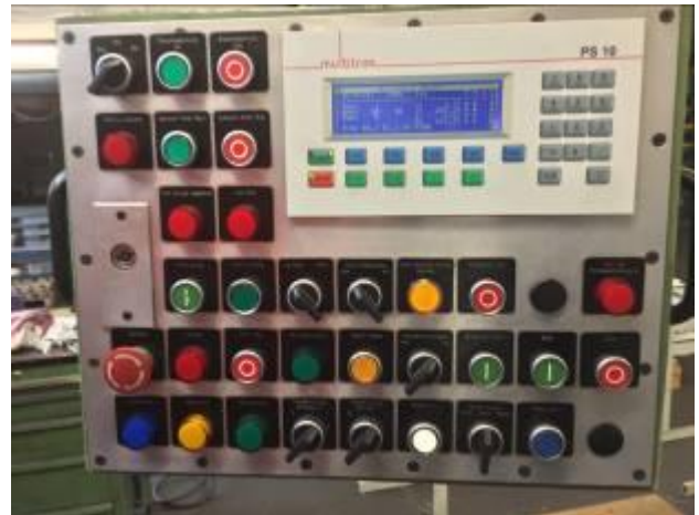
Figure 24: The CNC control with the operation was almost 20 years in operation.
