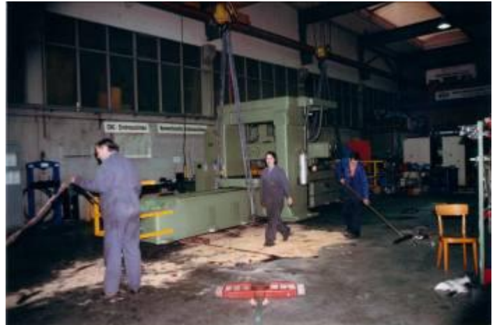
29: So now the machine is ready for lifting. In the middle Caroline Widmer, who then planned the whole electrical part and carried out.
