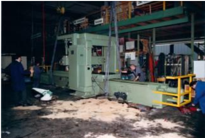
Figure 27: The Verlad the machine could be well performed with the 2 x 10 ton overhead cranes.
