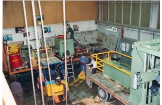
Figure 34: The remaining goods, including the large hydraulic unit is loaded onto the truck. Since several hundred liters of oil were there.
