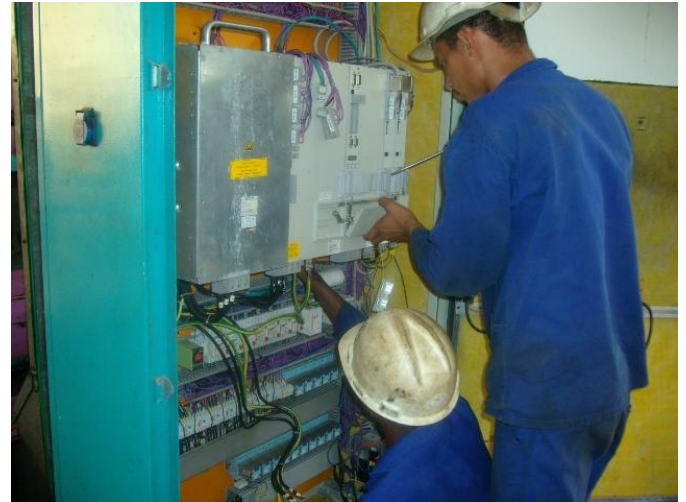
Figure 3: The entire spindle drive is replaced because there are no more spare parts warranty there was Siemens. And in Angola there now and have a blast. Here, tens of thousands of francs arising defects by the condensation that forms when one gets out a transformer power supply and several hours to cool the electrical cabinets. Now you have a standard engine taken 30 KW is less sensitive and a FU.
