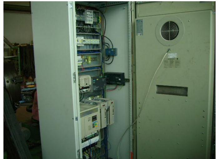
Figure 23: After Angola we only air-conditioned electrical cabinets. The worst is the condensation. When the plant is running, no problem there a power failure is, after about 8 hours, all full of water in the closet, and often it destroys the electronics. Also heaters are necessary when the temperature drops follows in the night and the day, the high humidity. The WIAP here has already invested many hours in studies for areas facing the sea in tropics. WU_260_150
